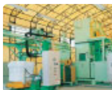
Waste compression and packaging plant
