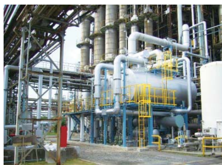
Cyclohexane recovery facility located within the Ube Chemical Factory premises
