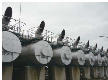
Deodorizing equipment at the Chiba Petrochemical Factory
