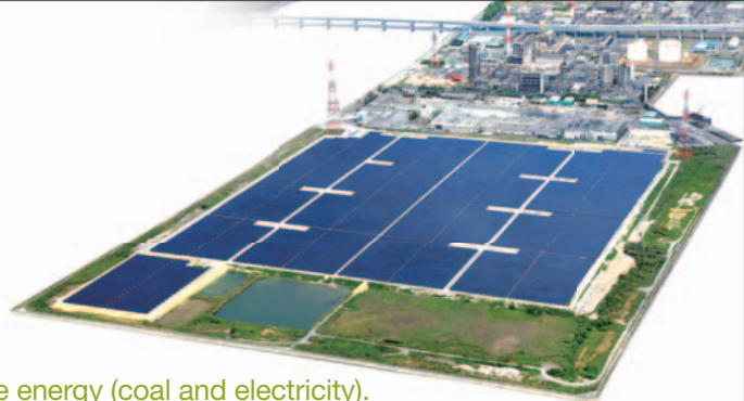
Solar power plant
