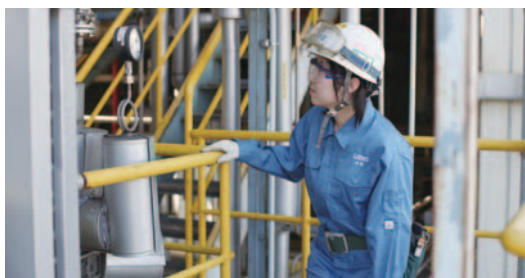
A female employee overseeing operating plant equipment at one of our factories
