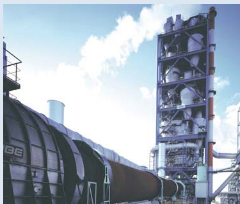
NSP kiln at Ube Cement Factory
